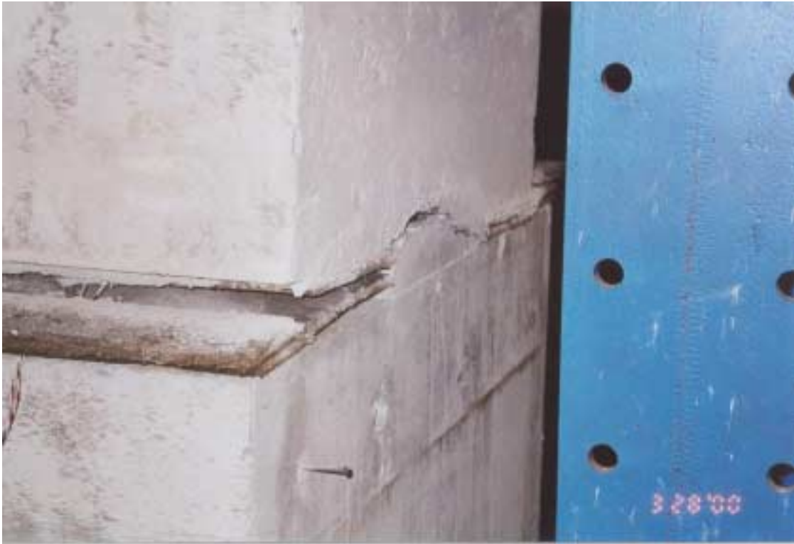
Figure 4.12. Picture of failed shear key
