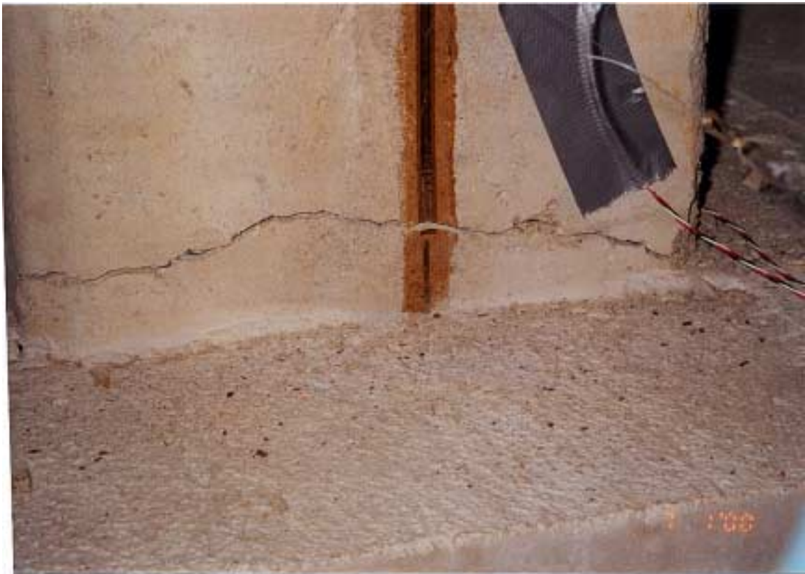
Figure 5.22. Pictures of the tension cracks developed in the first load cycle
