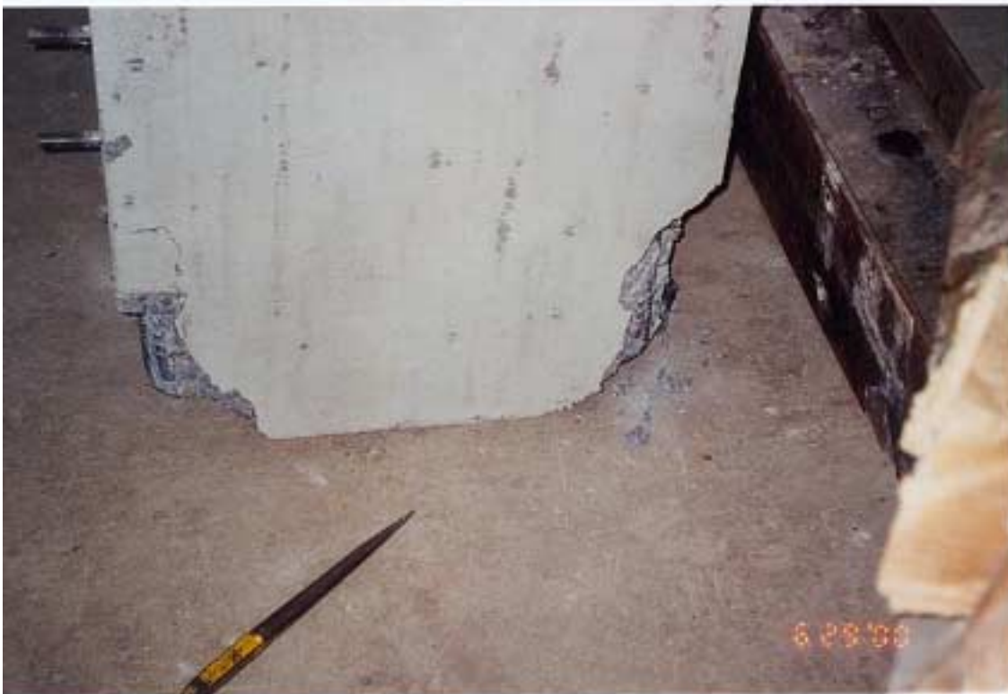
Figure 5.16. Pictures of the damage observed in the pile cap during testing
