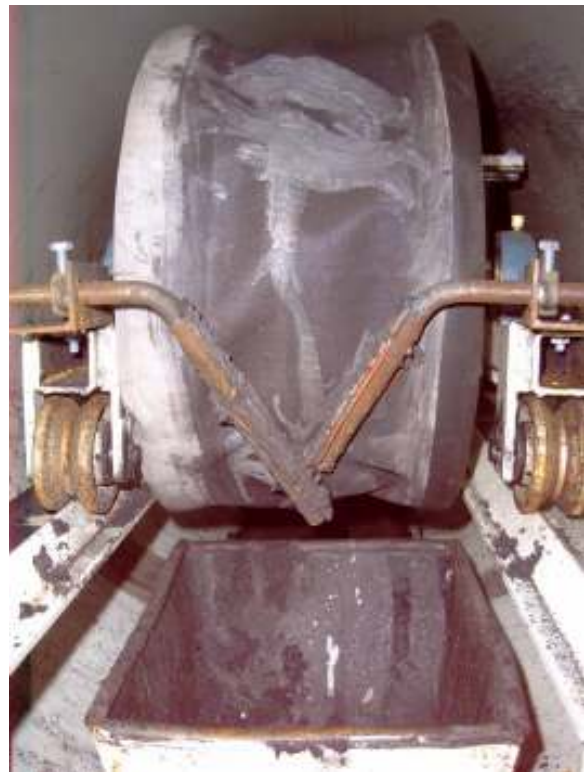
Figure 2.13. Scrapers used to remove fines from the filter cloth.
