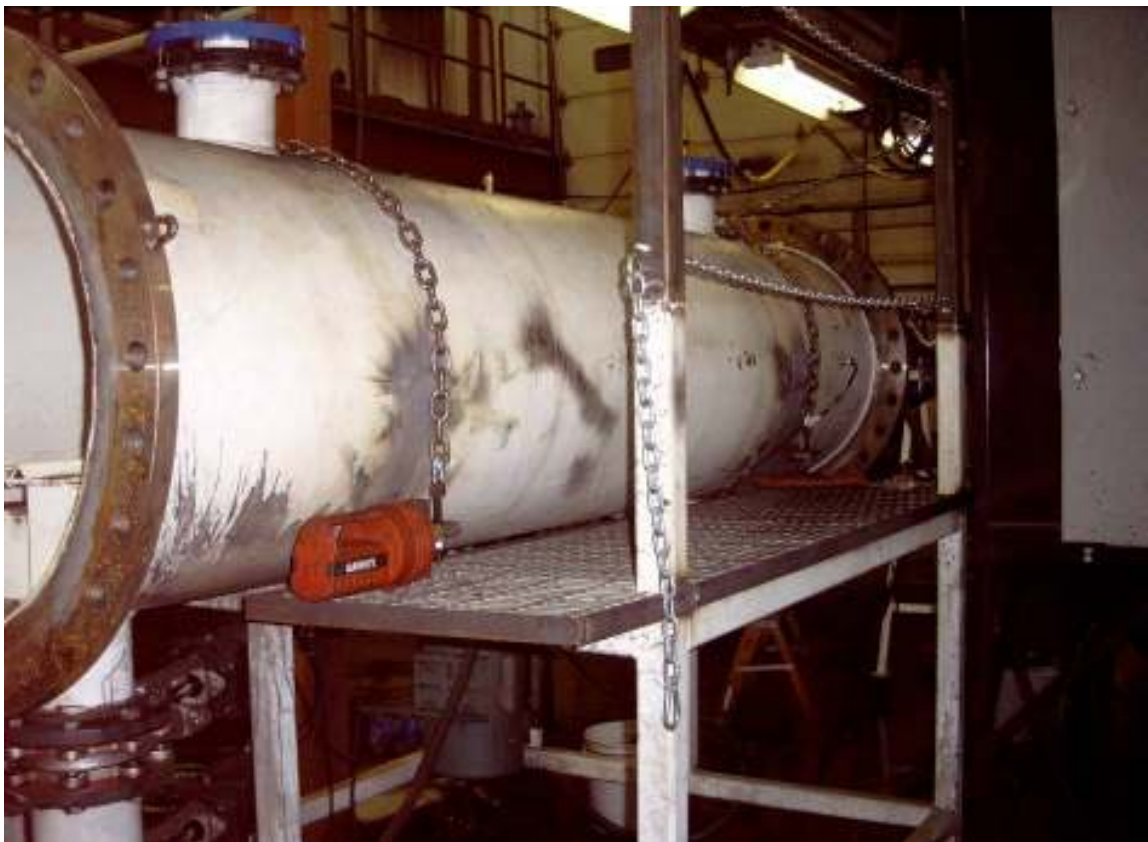
Figure 2.17. Walkway on the support frame.
