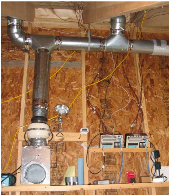
Figure 12. Interior side of the solar roof collector mock-up (wires from the sensors are connected with the two “Campbell Scientific, Model 21” data loggers)
