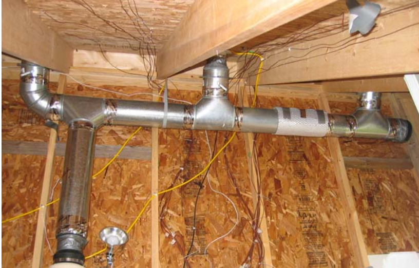
Figure 6. Interior side of the collector (The heated air is collected in the ductwork)
