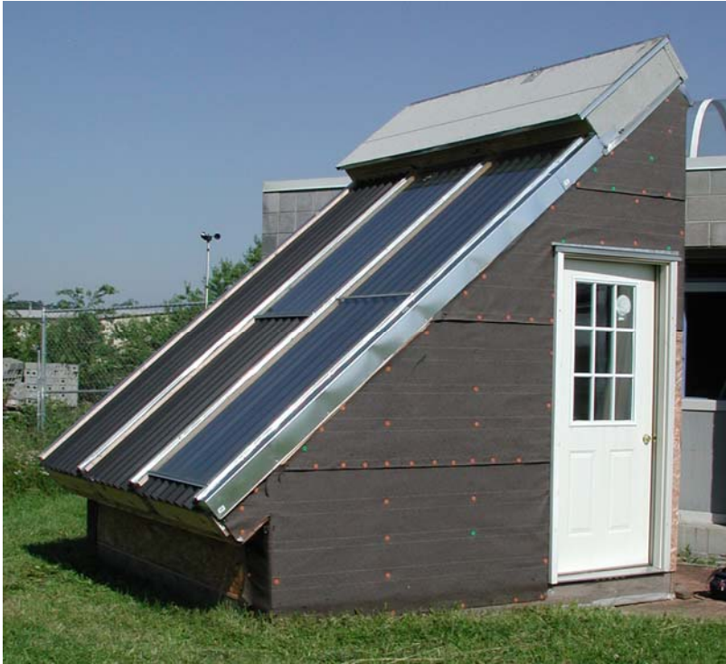
Figure 11. Southeast corner view of the solar roof collector
